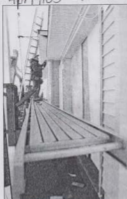
Dave LeBlanc attaches fascia recently to a new home at the south end of Riverview. The Town of Riverview is studying the possibility of setting up its own building inspection department.
