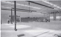
The bays in the new fire station give Riverview firefighters much more room.
