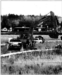
Enbridge crews work on the extension of the natural gas line to Riverview yesterday. The line will run parallel to the causeway, then run both east and west along Coverdale Road and possibly even up Pine Glen Road in work planned to be completed this fall.
